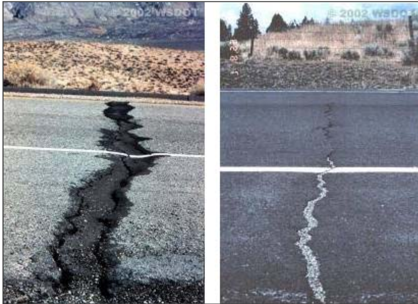
Figure 1 – Cracks from excessive pavement contraction.
